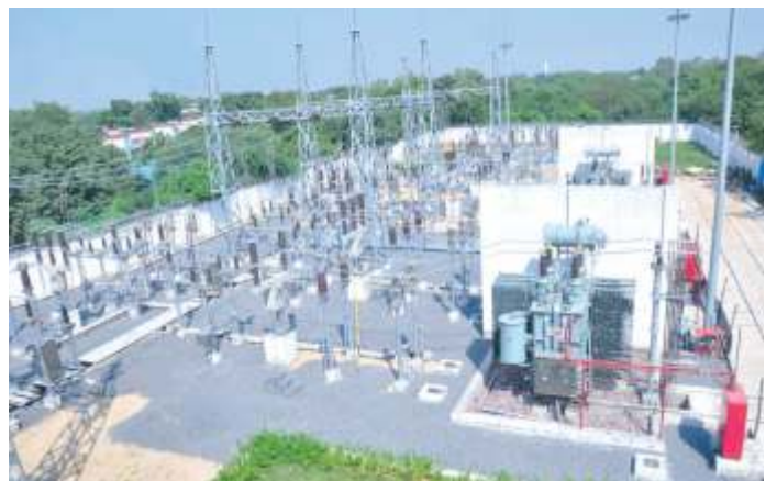
DMRC 66KV Sub Station at INA, Delhi
